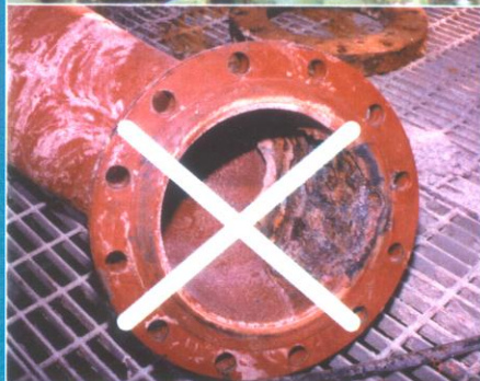
Dead Sea Works - Corroded steel elbow after 3 months of use.
